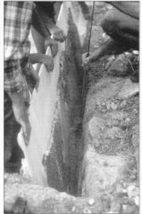
Figure 1 Detaching painted plaster that has remained attached to the stone footings of mudbrick walls at the Roman villa of Sette Finestre, Tuscany, Italy. The plaster has been protected with a cloth facing and as it is detached it is supported against a white board.
