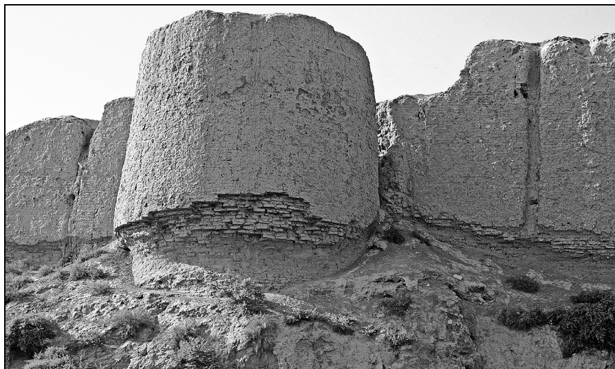
Figure 3 A corner tower of the Timurid city of Abdullah Khan Kala, built early in the fifteenth century AD, showing the erosion at the base of the walls caused by rising water and by the wind.
