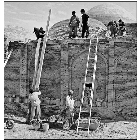
Figure 5 Repairing the roof of the mausoleum of Mohammed Ibn Zayd, a Shiite cleric. The concrete roof that had been added early in the twentieth century was too heavy for the structure and stopped it drying out when damp penetrated. It was therefore removed and replaced with a traditional earthen roof, which requires low maintenance and provides an effective weatherproof surface that allows the structure to breathe.
