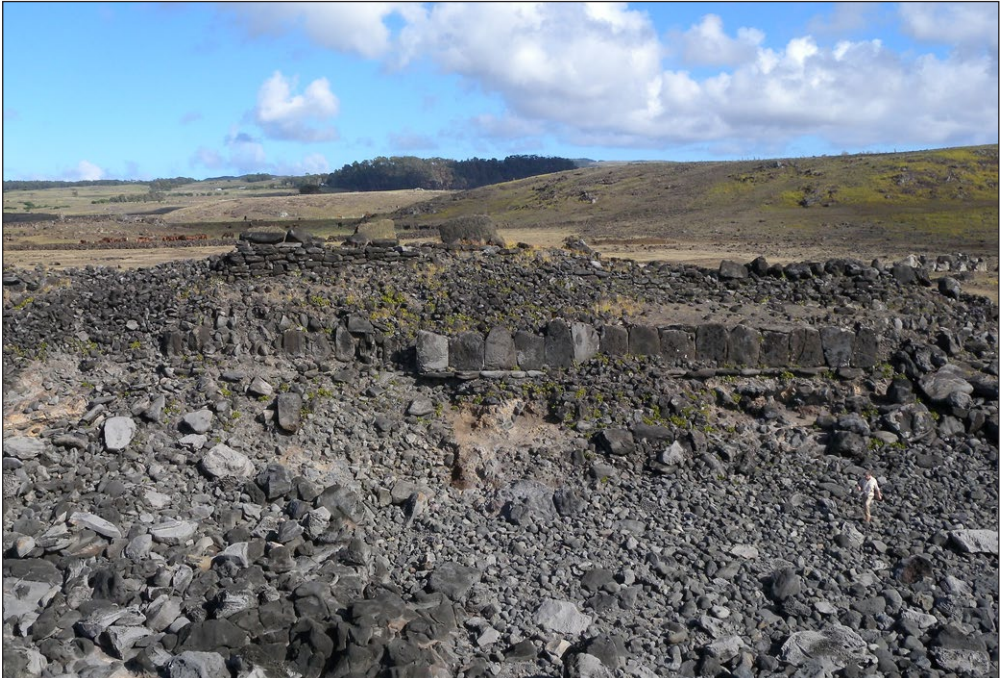
Figure 1: The rear of Ahu Ura Uraja Te Mahina, on the south coast of the Island. Sea erosion of the low cliff on which it stands has reached its rear wall, and is causing it to collapse (in the photo, the collapse is advancing from the left to the right). The bases of three prone moai are partially visible at the top of the surviving platform. Photo: Adam Stanford.
