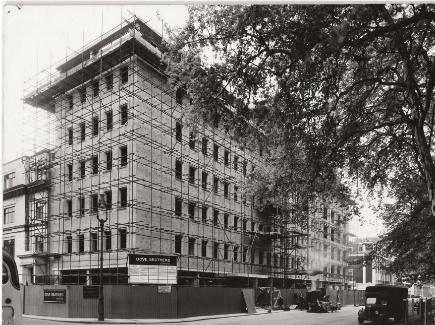
Fig. 1: Exterior view of the new Institute building as it nears completion in the mid 1950s. Despite the scaffolding and lack of window frames and glazing, the building is easily recognisable. Note the Dove Brothers' prominent sign.
