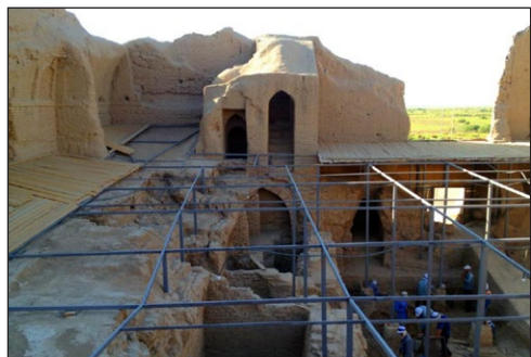
Figure 10: The supporting arch of the ground floor barrel-vaulted rooms, visible below the staircase (Photograph Rejep Jepbarov).
