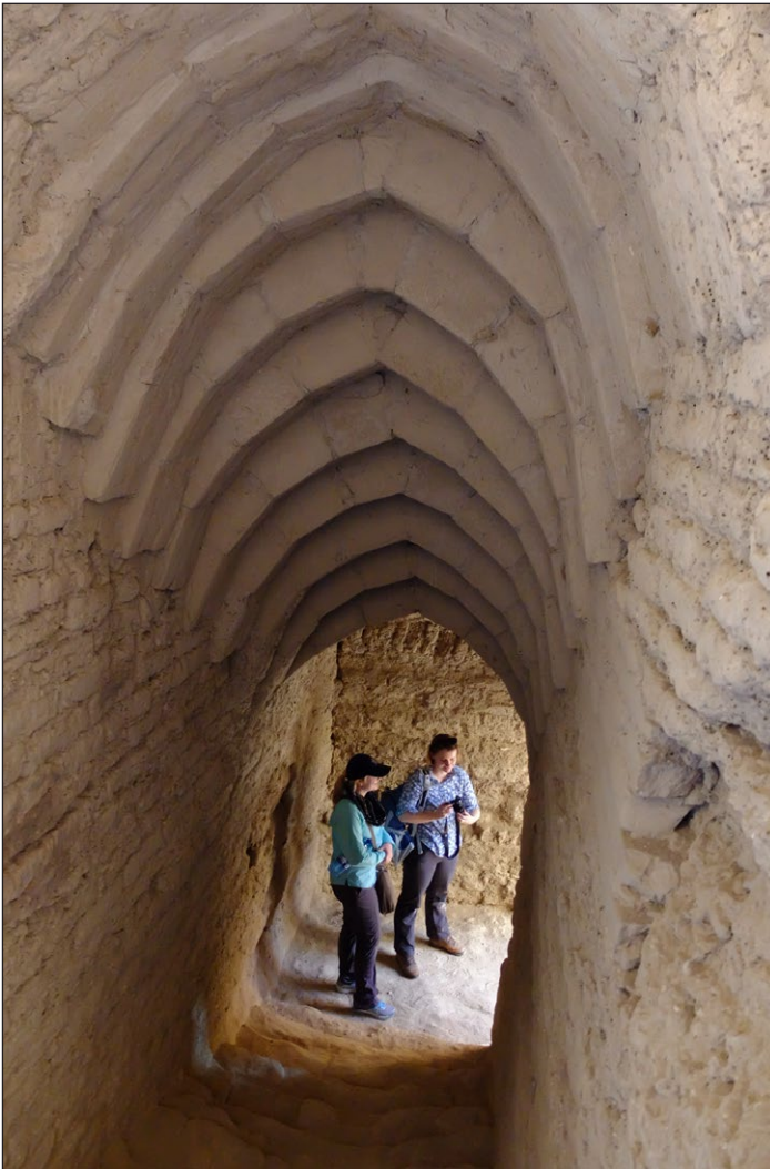
Figure 13: Internal staircase, roofed by a series of stepped tunnel vaults, leading down from second storey to the courtyard (Photograph Sébastien Moriset).
