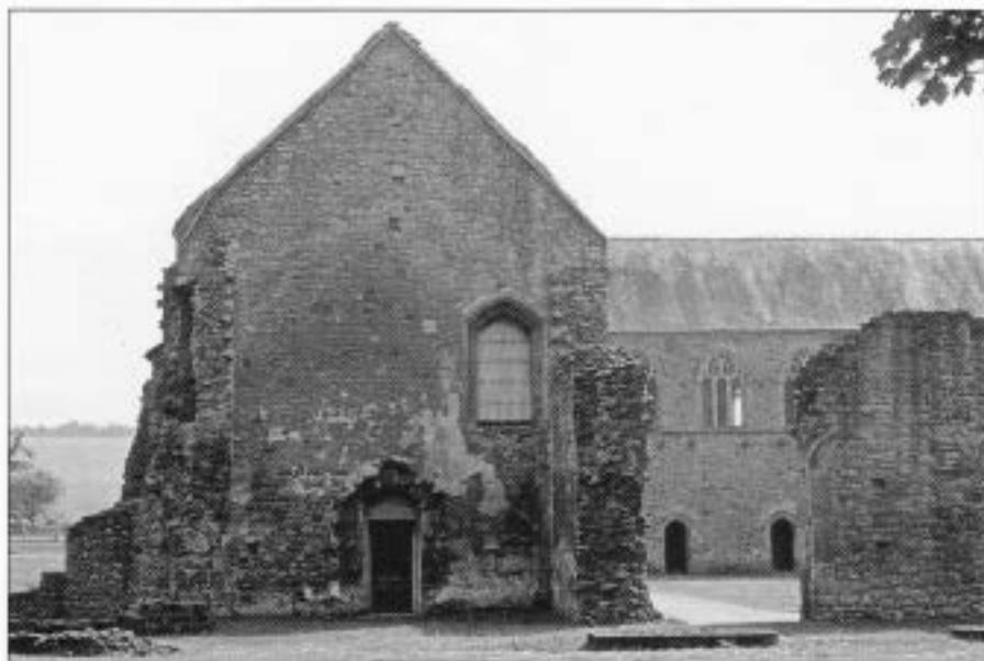
Figure 4 Cleve Abbey, Somerset: the exterior of the sacristy and cloister viewed from the north, 1998.
