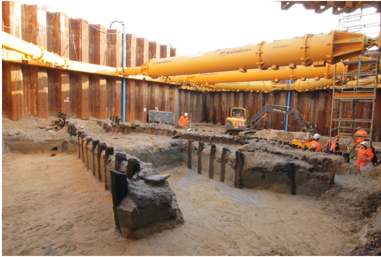
Figure 10 Excavating the wooden remains of the Elizabethan harbour at Dover Western Docks, Kent (Source: ASE)
