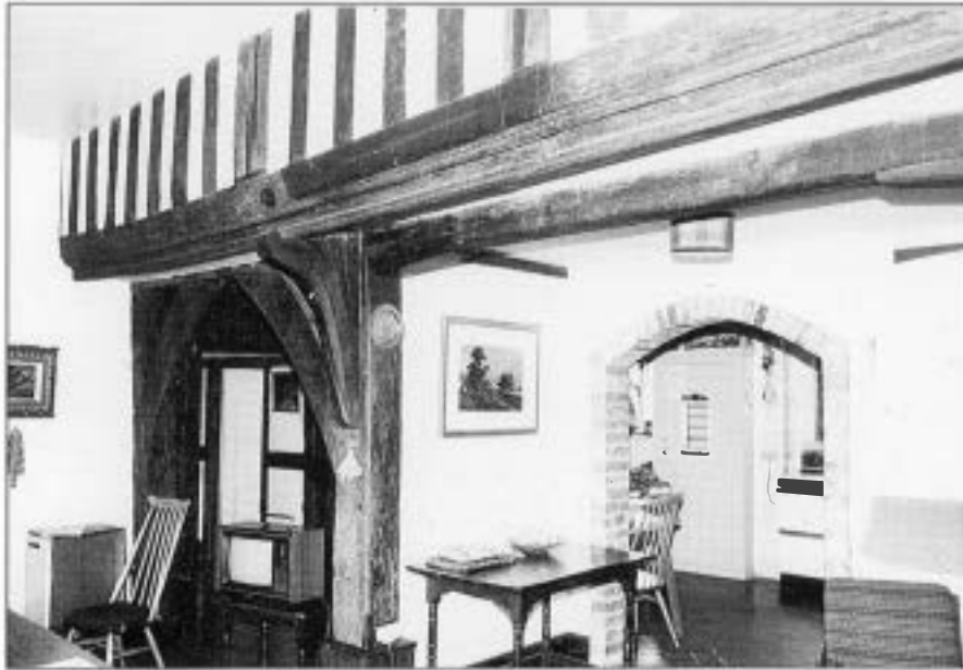
Figure 4 The original southern external wall (upper left) of the kitchen at Comphurst, now visible within a later addition. The ground-floor section of the external wall has been removed, but mortices in the remaining timbers provide evidence of its design.
