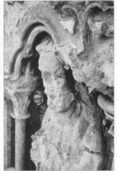
Figure 2 Decayed apostle, Wells Cathedral. The limestone reacts with acidic air pollutants to give salts, which then cause further damage.
