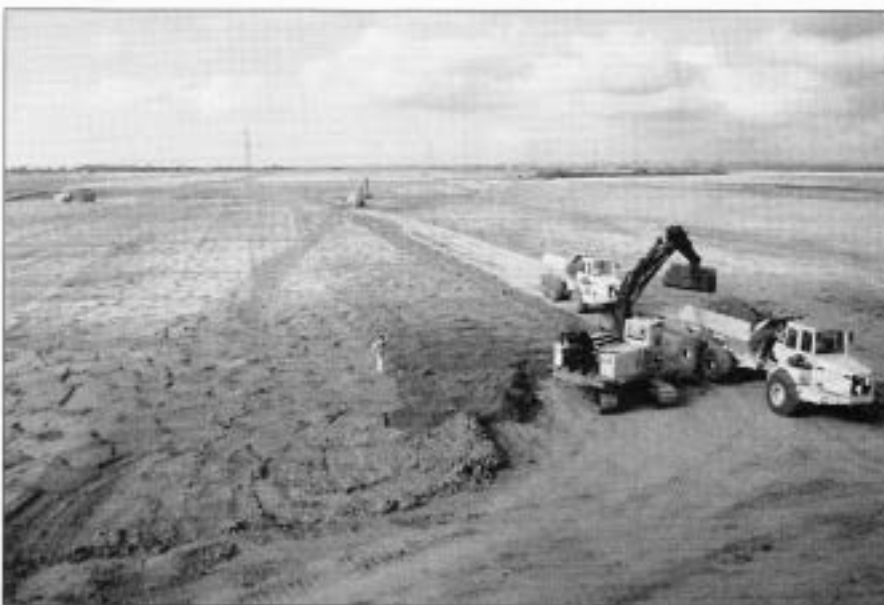
Figure 4 Stripping topsoil during the first phase of excavation (Lydd 1) at Lydd Quarry.
