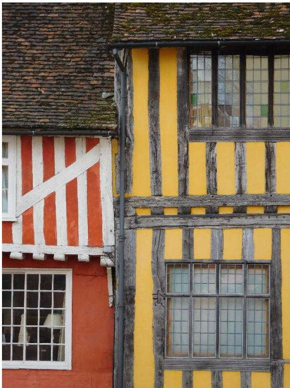
Figure 1. C15th timber framing, The Manor House (left) and 53 Church Street (right), Lavenham, Suffolk. Source: (Whitman, 2017)
