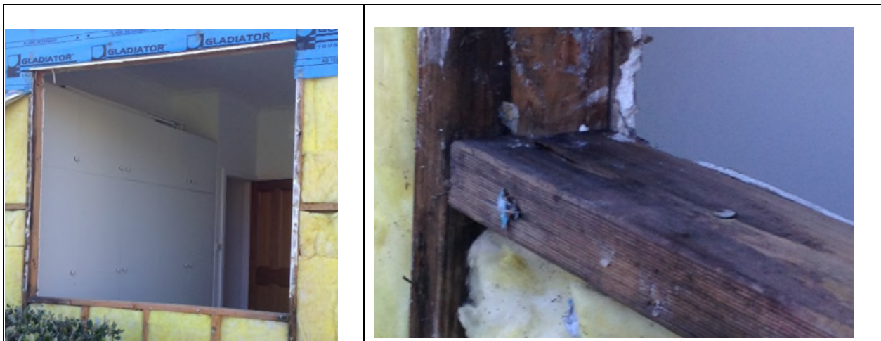
Fig. 3: Example of moisture ingress causing degradation of timber framing in Australian residential construction
