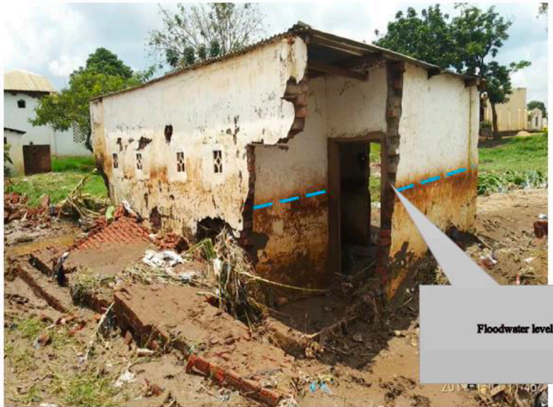
Figure 4a: Flood water level inside and outside a damaged house
